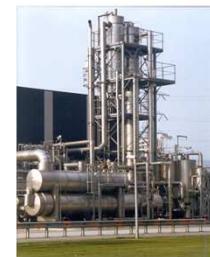
Distillation column of a CO 2 liquefier
